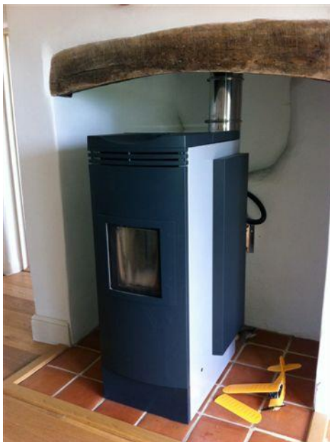
Biomass boiler in a rural farmhouse
